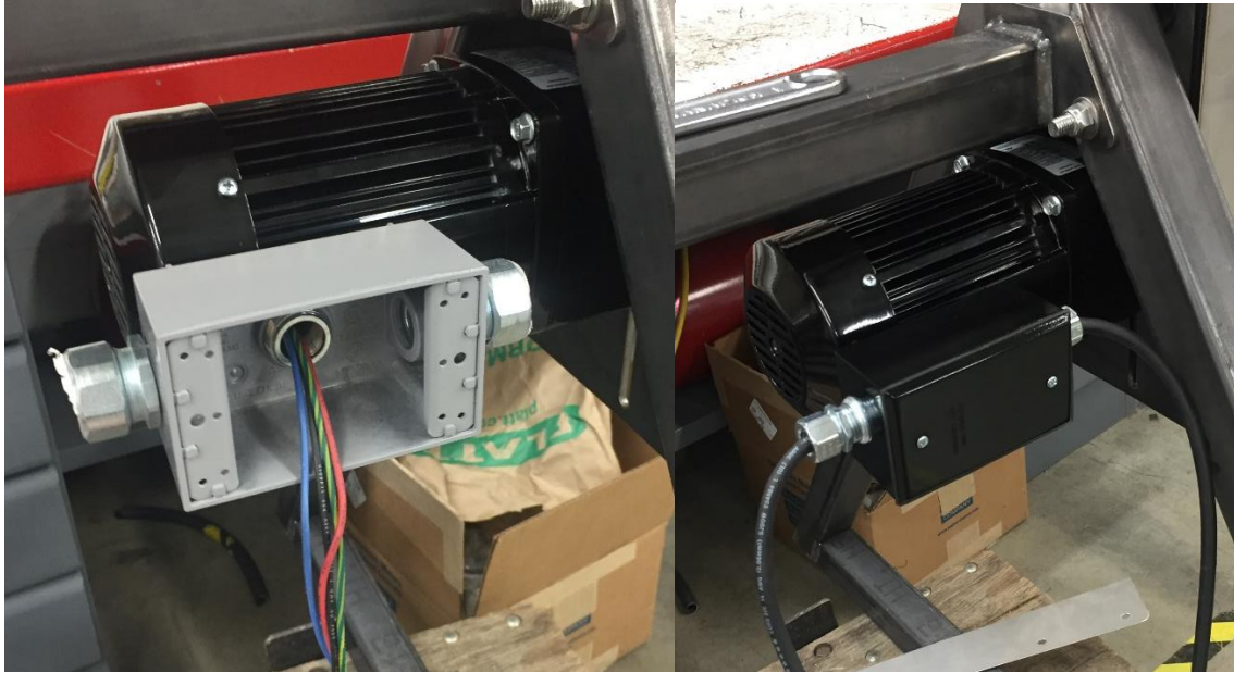
Figure 8: Electrical Box before and after
