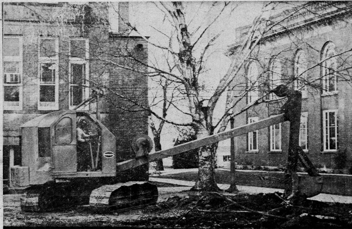
TIMBER! TREES, BUSHES AND SHRUBS fell under the constant energy of workmen clearing the east side of the Classroom building. The work is being done to clear the way for the addition to the building, which was originally constructed in 1929. Three rooms and a fire escape will be added. The work is scheduled to be completed this year.
