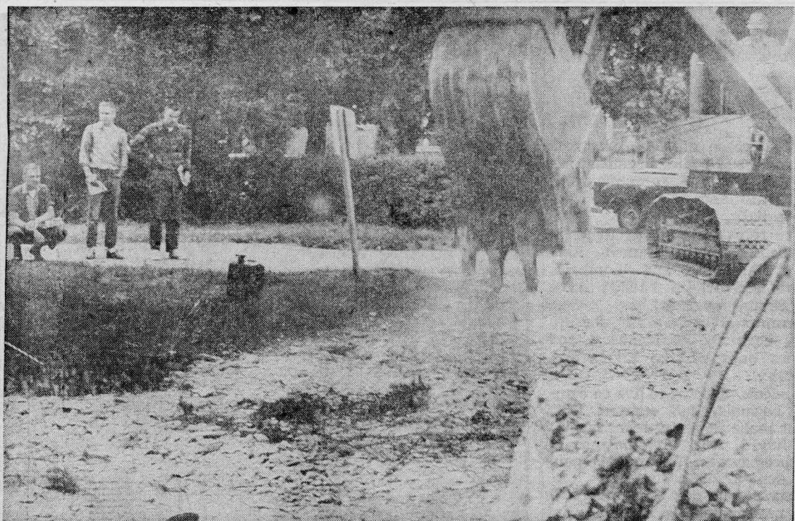
CWC SIDEWALK SUPERINTENDENTS Dick Lowe, Tom Reeder and Jerry Murphy stop to supervise the steamshovel at work outside the front of the CUB. Men are at work tearing up the street to make way for the development of a plaza on 9th street. Work on the plaza must be finished by July 1 so improvements were started at this time. The street will be completely torn out and benches will be built around trees for student convenience. (Photo by Bill Craig)
