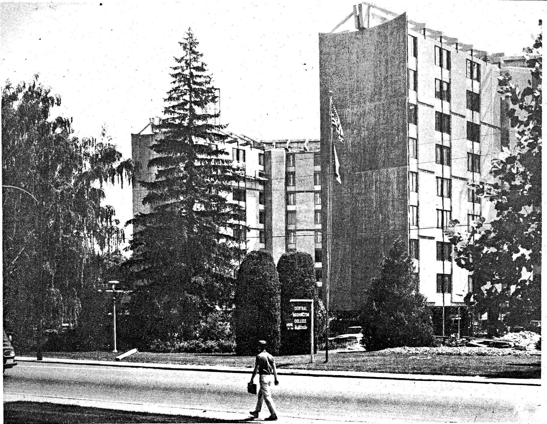
RACE THE CLOCK—The nine-story high rise dormitories, newest addition to Central's growing campus, loom behind the Central sign appearing as if they are an additional welcome for new and former students this fall. A meeting this Monday between the construction
