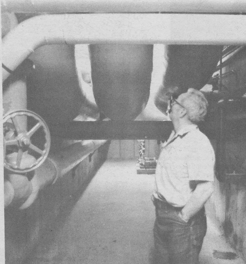
STEAMY MAMMOTHS —Bob Lahey, physical plant, must make safety checks on the large boiler tanks and pipes. (Photo by Mary Wallace)
