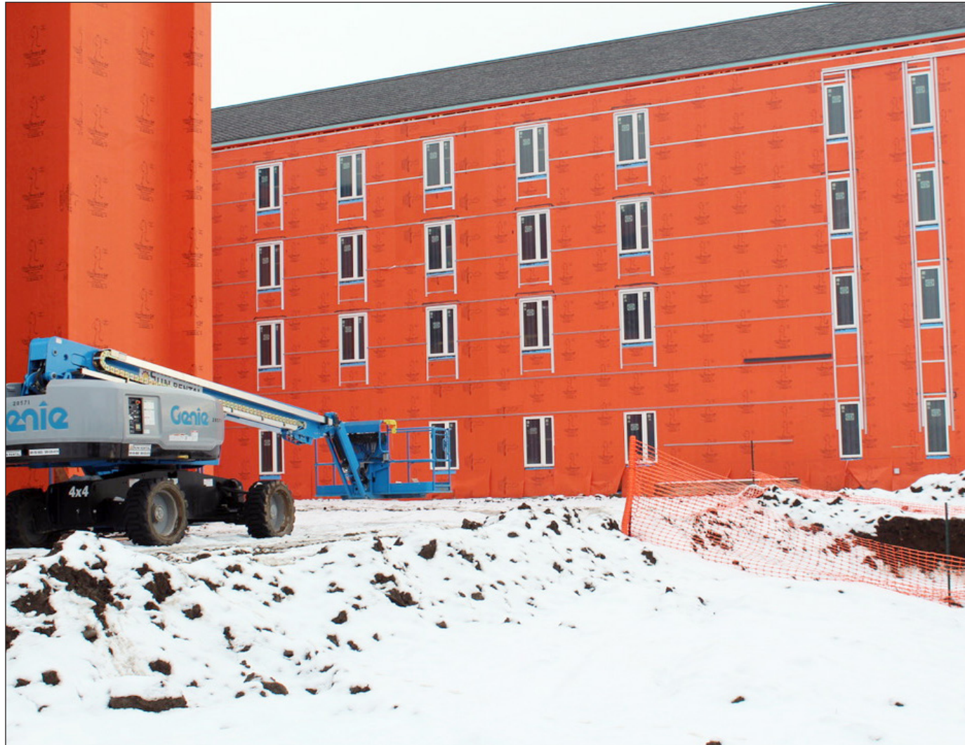
Dugmore Hall is currently undergoing construction on a budget of $40 million. The project is the first time CWU is using a progressive design build, that will allow the university to work closer with Lydig Construction and Mahlum Architecture. Heather Stewart/The Observer
